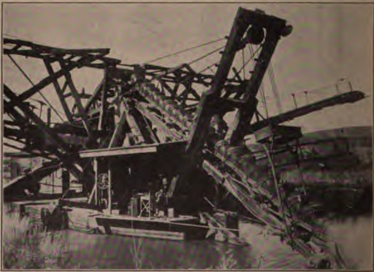
View of Excavating End of Ladder Dredge on Irrigation Work in Washington.
